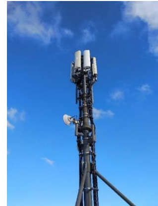
Figure 1. Example of antenna support on a roof.
